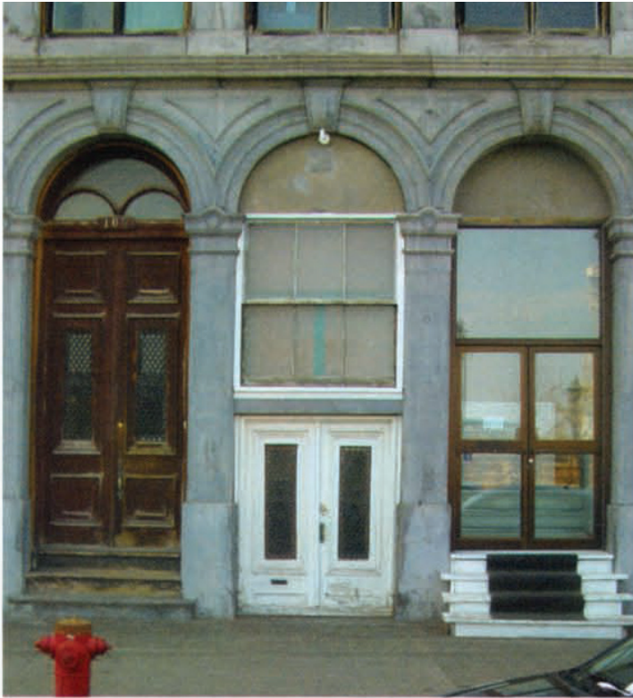
Windows are not the only elements maligned by inappropriate replacements.
