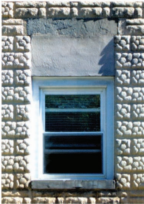
The window replacement resulted in reduced visibility and daylight.
