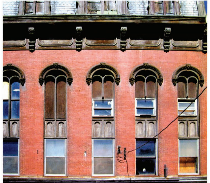
The damage wrought by replacement windows is self-evident and increasingly pervasive. All photos: © Walter Sedovic Architects.
